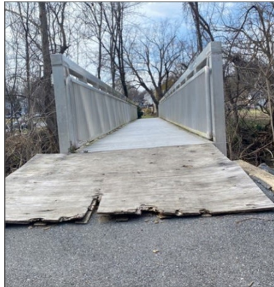
Figure 25. A bridge crosses Sligo Creek on the north side of MD 410 (East West Highway). (PHOTO BY TOOLE DESIGN GROUP)
