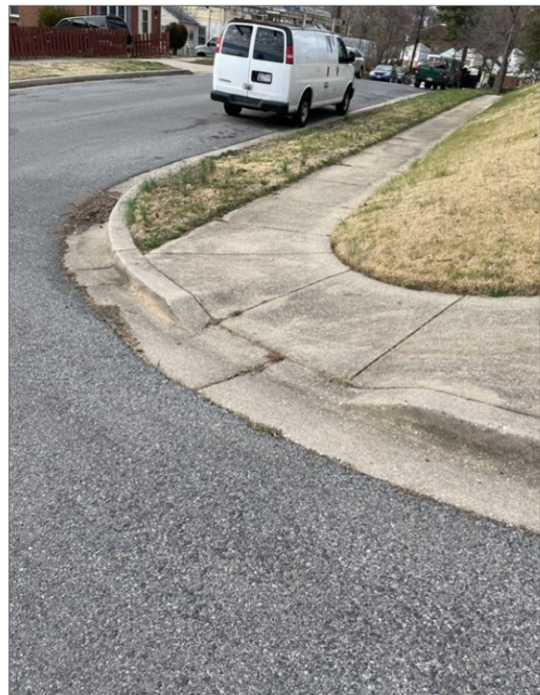
Figure 12. A curb ramp at 17th Avenue and Amherst Road has no detectable warning surface. (PHOTO BY TOOLE DESIGN GROUP)
