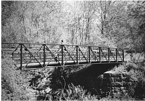
Pedestrian bridges over Paint Branch will provide convenient connections between The University of Maryland campus and the US 1 corridor.
