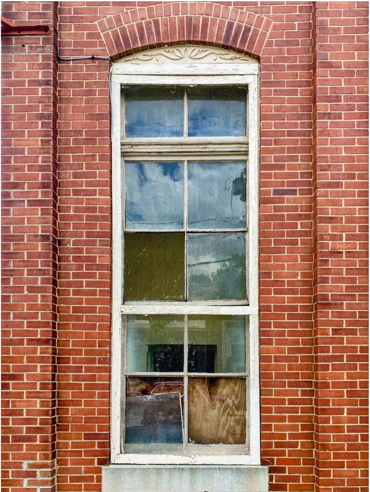
Figure 19. Detail of the northeast front window at the Mount Hermon Masonic Temple, May 11, 2024.
