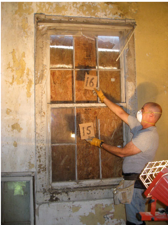
Window "A" from interior, north elevation, showing damaged and missing muntins in both sash which will be recreated.
