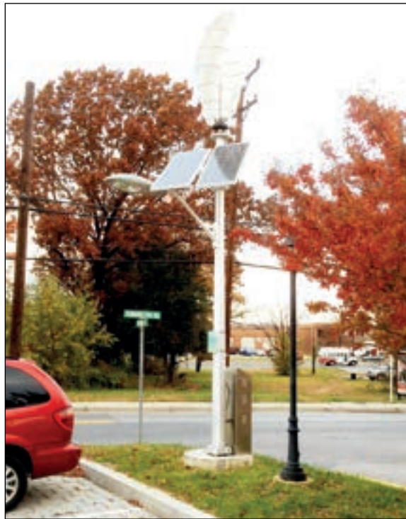
Parking Lot Lighting with Solar Panel and Wind Turbine
