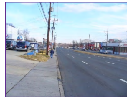
Driveway with steep cross-slope along University Boulevard (MD 193)
