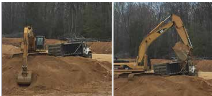
Figure 1. Photograph illustrating sand and gravel mining operation in progress, southern Prince George's County, 2018.
