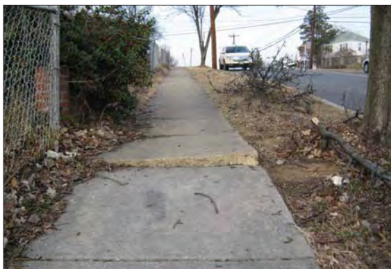
The tree's roots have caused this sidewalk to bulge creating a tripping hazard and barrier for wheel-chair users.
