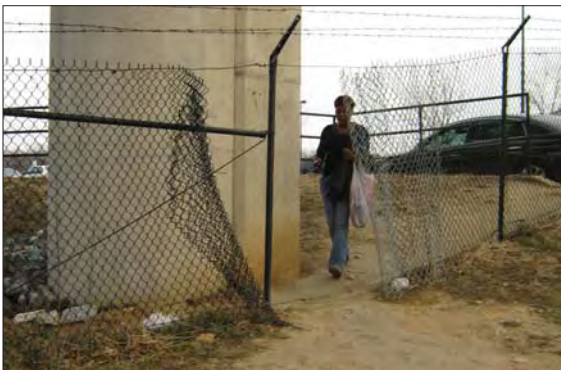
This fence around the Naylor Road Metro station is located at a natural pedestrian access point and has been repeatedly cut open and repaired.
