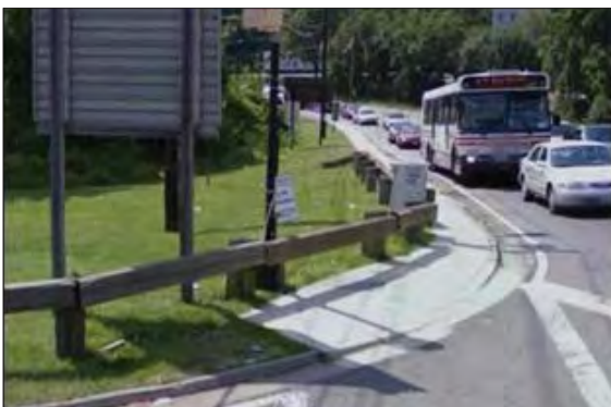
Pedestrian signal heads at the intersection of Suitland Parkway/Naylor Road are either missing or misplaced.
