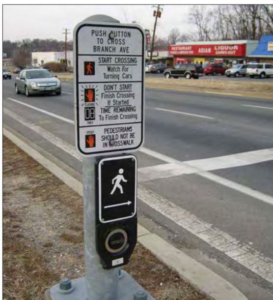
A pedestrian push-button is provided to cross Branch Avenue at Naylor Road. Actuation demonstrates that pedestrians have been planned for, and this type of button provides audible feedback to the user. However, automatic pedestrian signals reduce delay for pedestrians.
