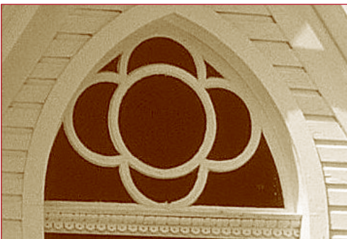
Detail of a quatrefoil overdoor window at the Holy Family Roman Catholic Church.
