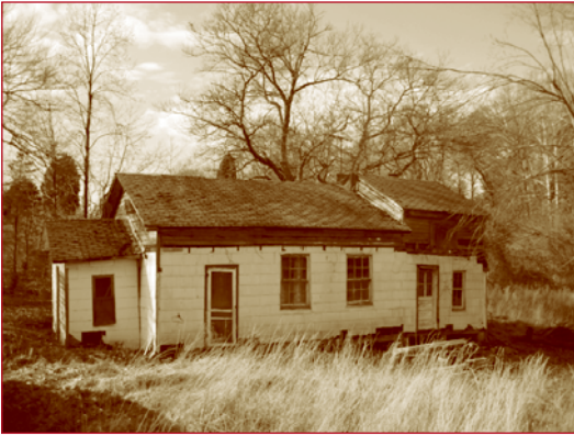
The Black Swamp School near Aquasco, prior to its restoration. The one-and-a-half story addition (now demolished) was added by the Daniel Skinner family after they purchased it for use as a residence in 1936.
