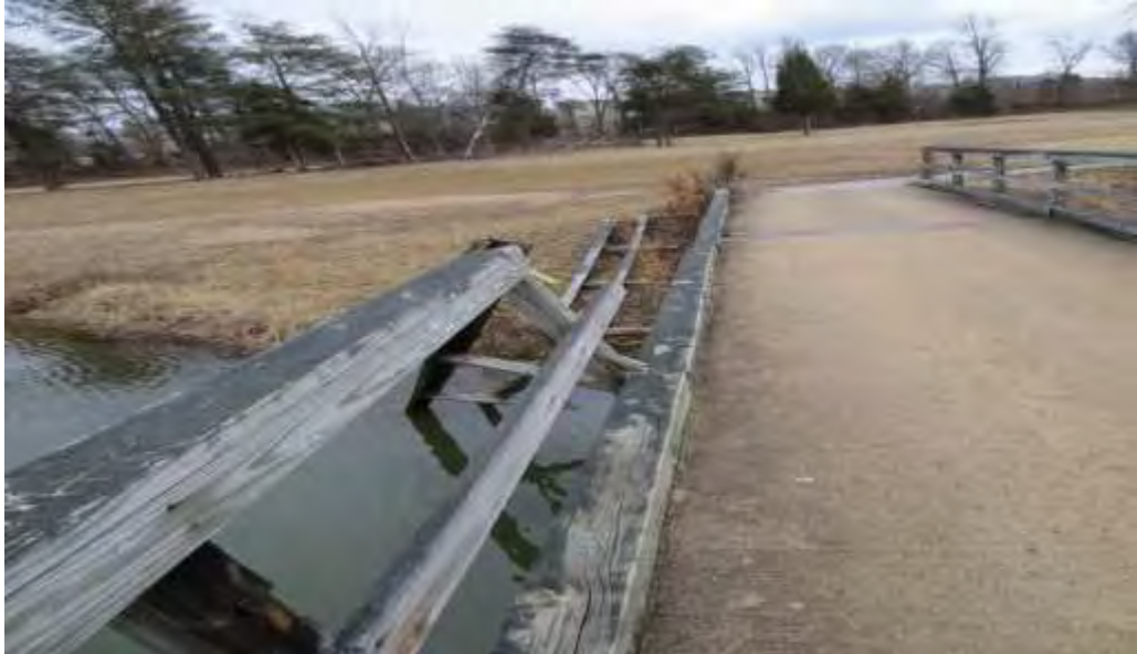
Collapsed bridge railing.
