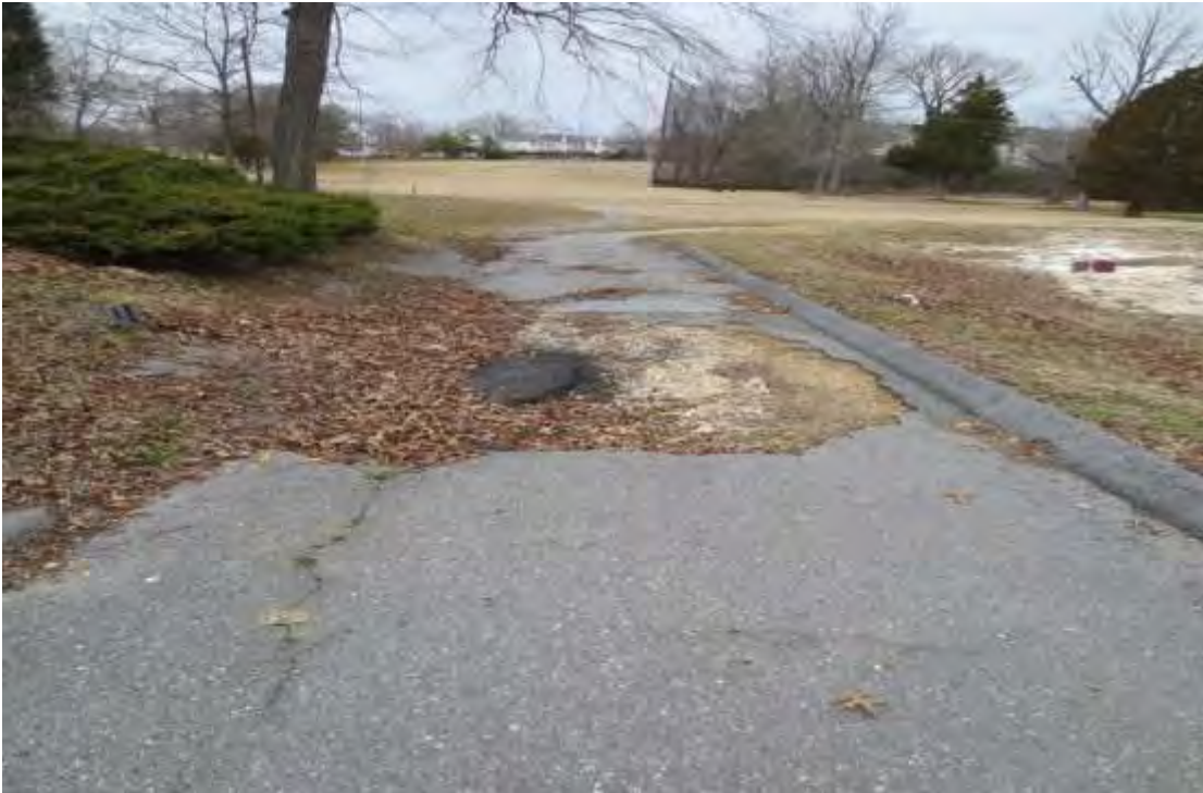
Deteriorated cart path.
