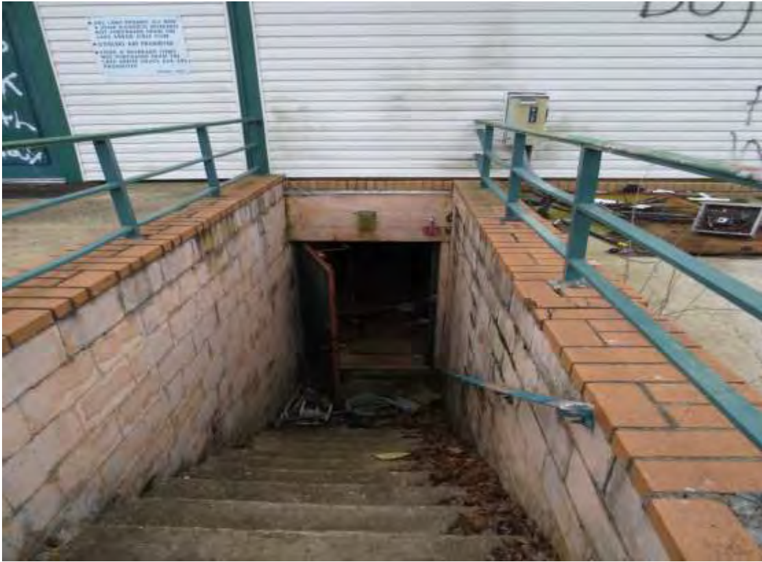
Unsecured entrance at the Club House.
