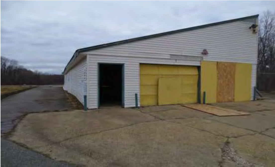
Unsecured entrance to the golf cart shed.
