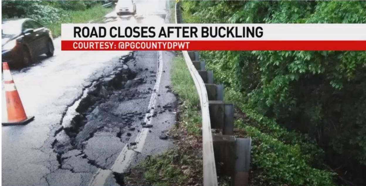
Figure 5 – Potholes Developing after Flooding Fort Washington MD
