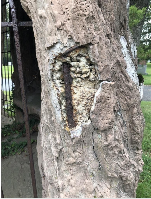
Photo 22: Hollow Tree Sculpture, damaged area where the outer concrete layer has fallen away, revealing the concrete and rebar underneath. The exposed rebar has begun to rust. Photo Source: Photograph taken by PALS Research Team
