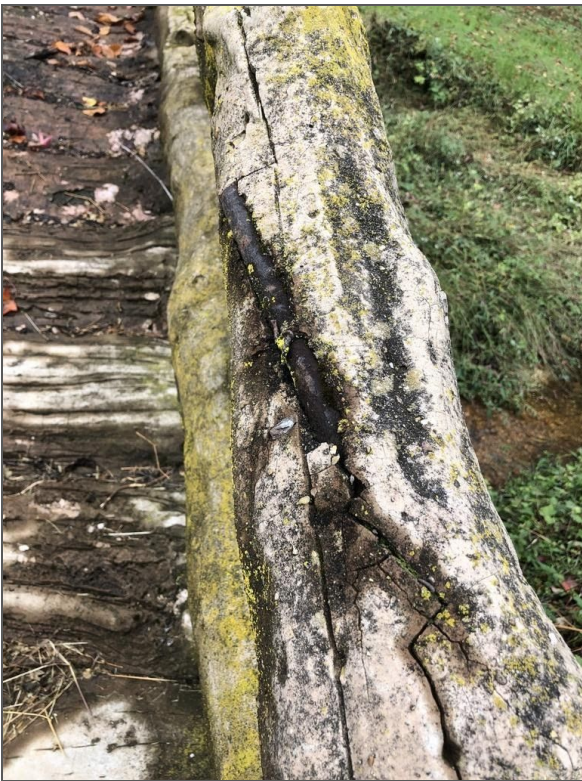
Photo 33: These various problems are common to many of the sculptures, including cracking and breaking off of the outer layer of highly cementitious concrete, the exposure of rebar, and biological growth
