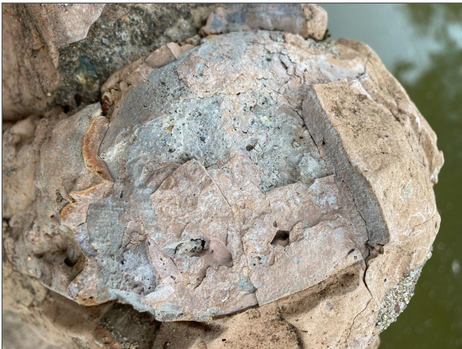
Photo 14: Spalled or debonded broken outer concrete layer revealing the base concrete layer Photo Source: Photograph taken by PALS Research Team
