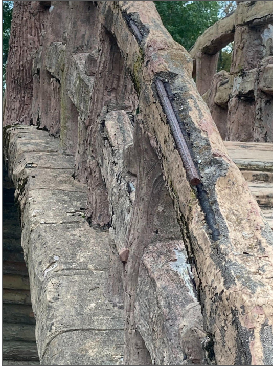
Photo 13: Exposed rebar and metal lath on the Bridge of Life, Cedar Hill Cemetery Photo Source: Photograph taken by PALS Research Team
