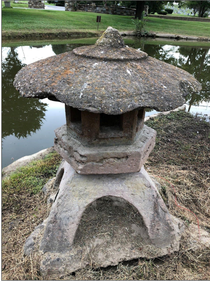
Photo 18: Lantern 2, areas where concrete has chipped off Photo Source: Photograph taken by PALS Research Team
