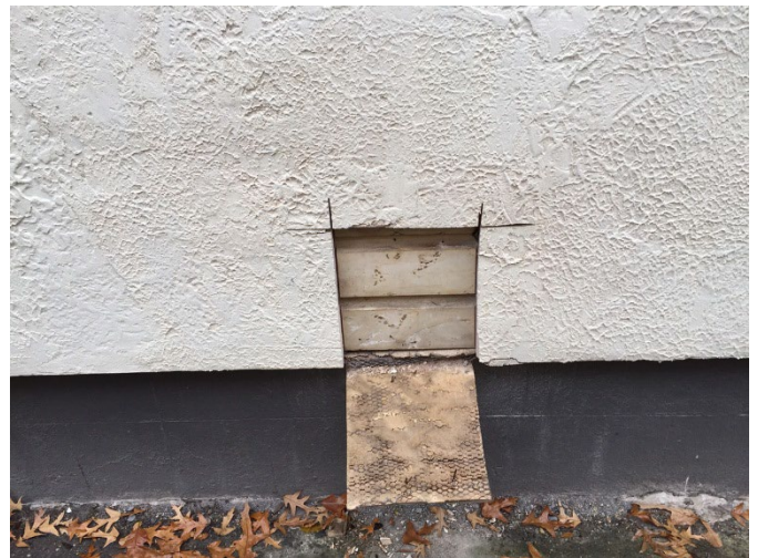
East elevation. Portion of stucco removed to show original drop siding underneath, which will be restored.
